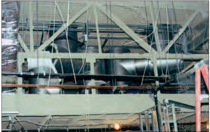
Space was tight, especially in the mechanical mezzanine above the original kitchen area.
